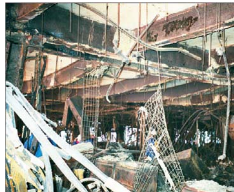
Figure 2-5 Deformed Floor Beams post Fire in WTC 5 (FEMA 403)
