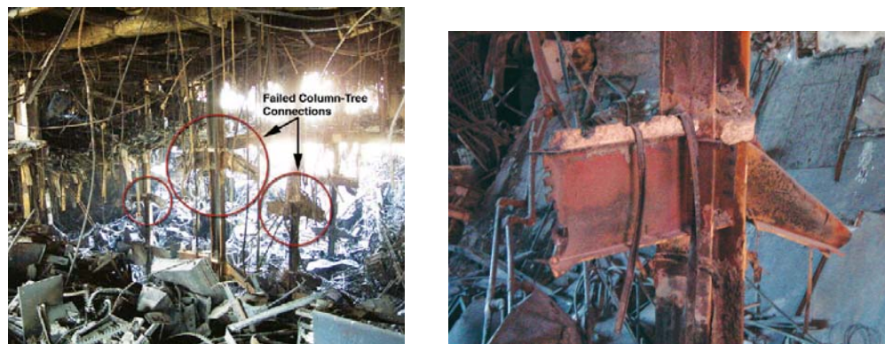
Figure 2-7 Failed Column Tress Connections in WTC 5 (FEMA 403)
