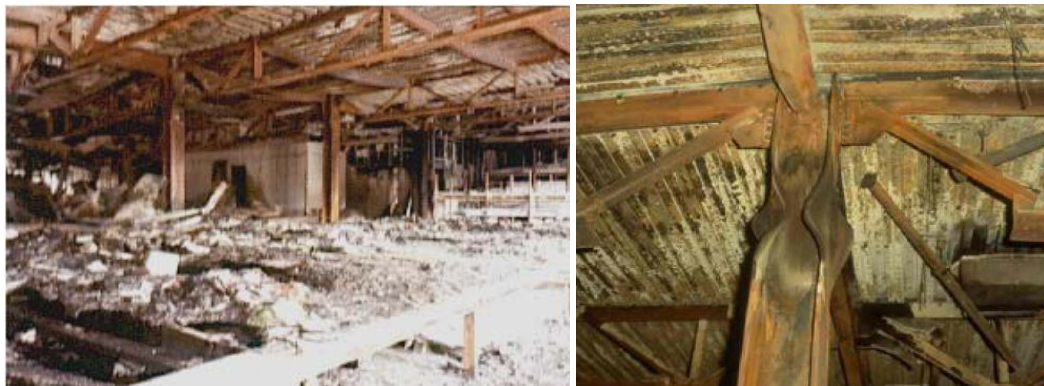
Figure 2-2 Broadgate Building and local buckled column after Fire (Ivan Burgess, 2002)
