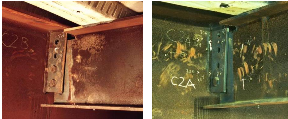
Figure 2-14 Connection Failed in Fire (left) and in Cooling Phase (right) (Cardington Fire Test Report, 1998)
